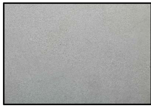
6. CONCRETE PERMEABLE PAVERS ON DRIVEWAY
